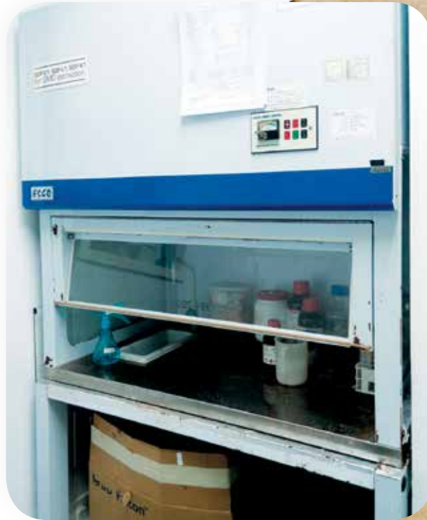
18 year-old Ductless Fume Hood HONG KONG
